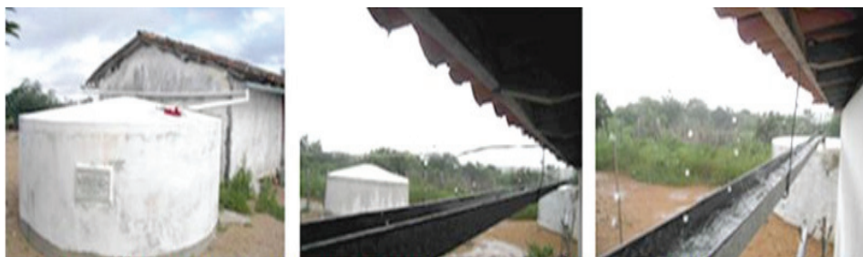
Figure 4 – Cistern and the capture of rainwater
