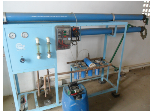
Figure 3 – Desalinator, Community of Encruzilhada Ferreiras- PE
