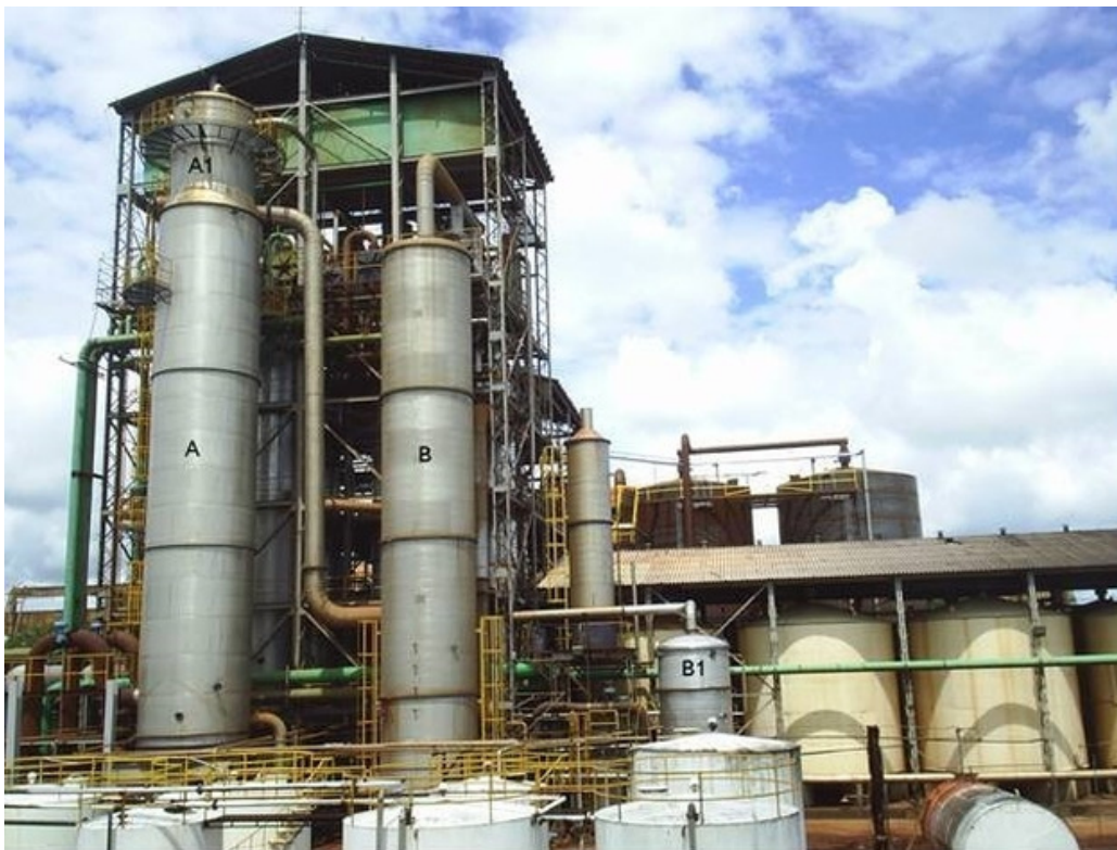
Figure 2. Distillation Columns of the industrial plant of COCAFÉ.
