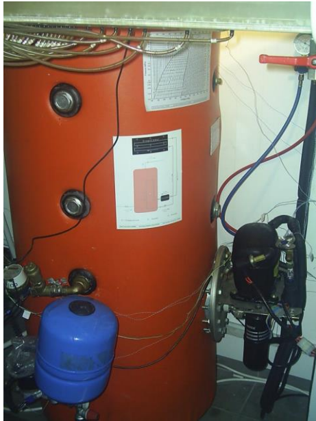
Figure 2: Thermal storage tank and compressor
